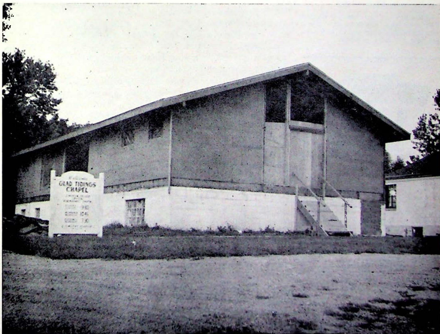
GLAD TIDINGS CHAPEL, Dayton, Ohio, which has received assistance from the Mission Builder's League is now under construction and will soon be completed and ready for use.
