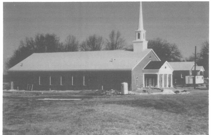
The new sanctuary for the Guthrie Grove Church of God, Pelzer, SC. This church will receive the Fall 1992 Church Builder's Appeal.
